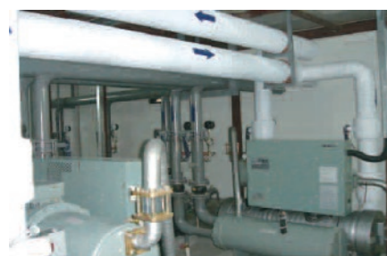
Machine Room for Conventional Central Water-source Unit
